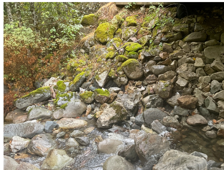
Downstream right bank riprap erosion
