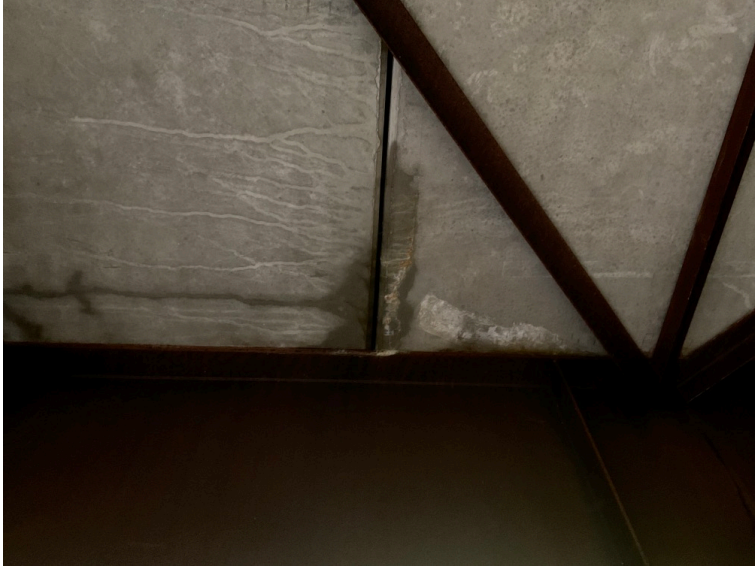
Panel 2 on left bank, efflorescence
