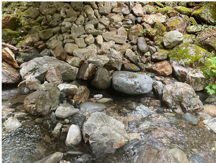
Erosion noted on left bank riprap
